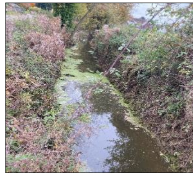
A maintained channel that will allow flow to pass, without removing all vegetation.
